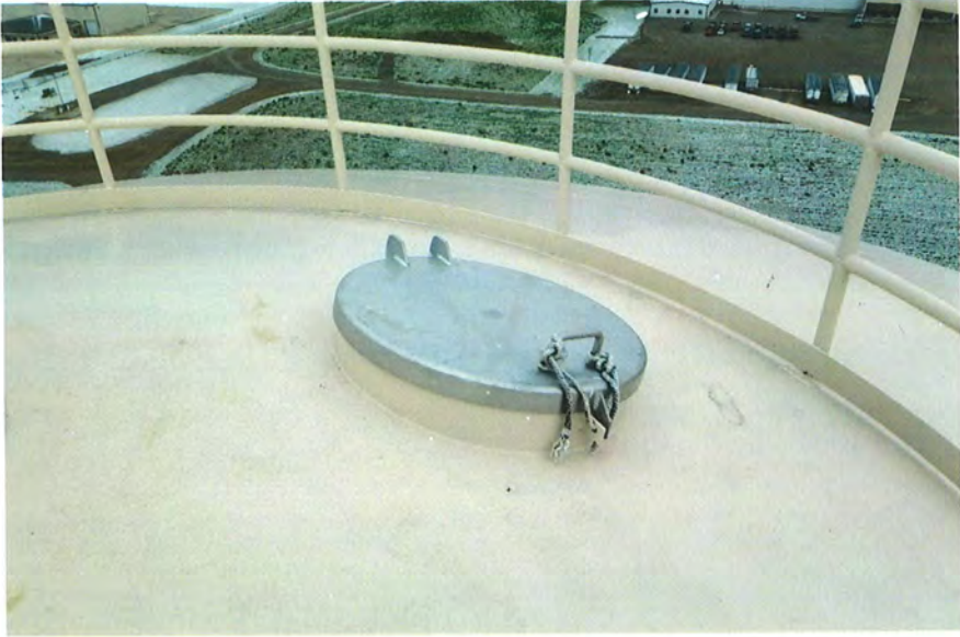
Roof access hatches are in excellent condition and operate freely. The aircraft warning light also appears to be in great condition.
